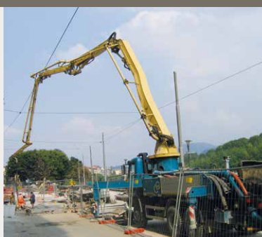
Pompaggio CLS alleggerito a base di Pomical / Pumping of lightened concrete having as basis Pomical
